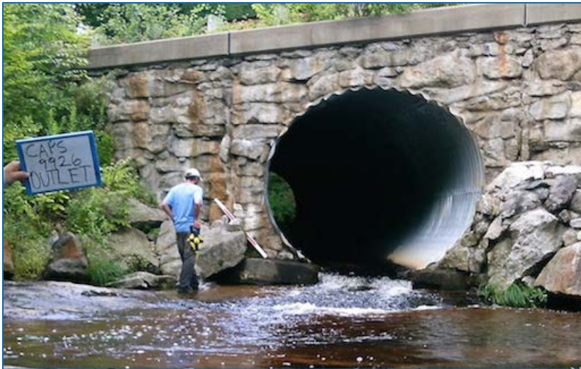
Figure H-5: Culvert 9926 inlet (top) and outlet (bottom) with a diameter of 10 ft on both sides.
