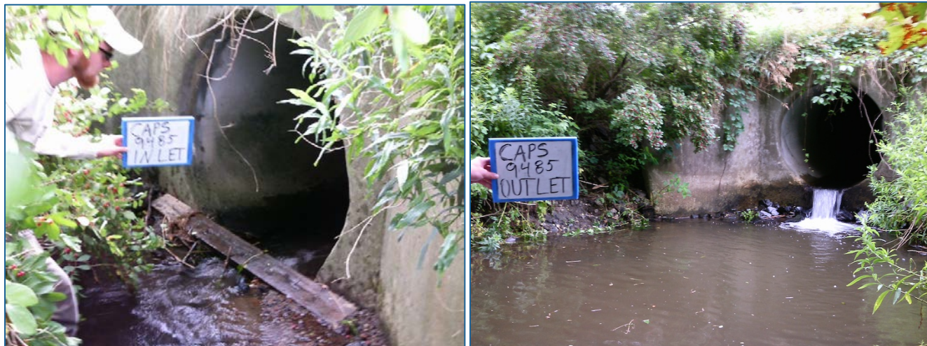
Figure H-3: Culvert 9485 inlet and outlet. The inlet (left) has a diameter of 4.5 ft. The outlet (right) has a diameter of 5 ft.
